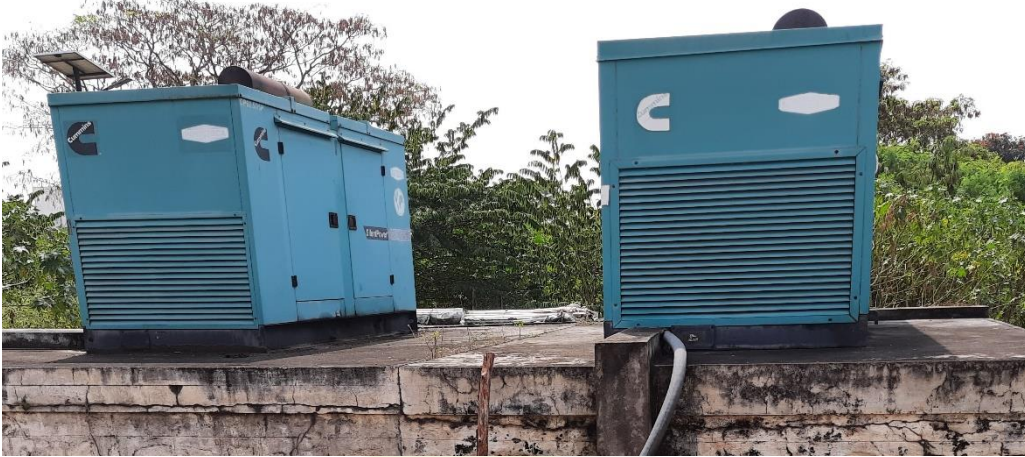
College Diesel Generator
