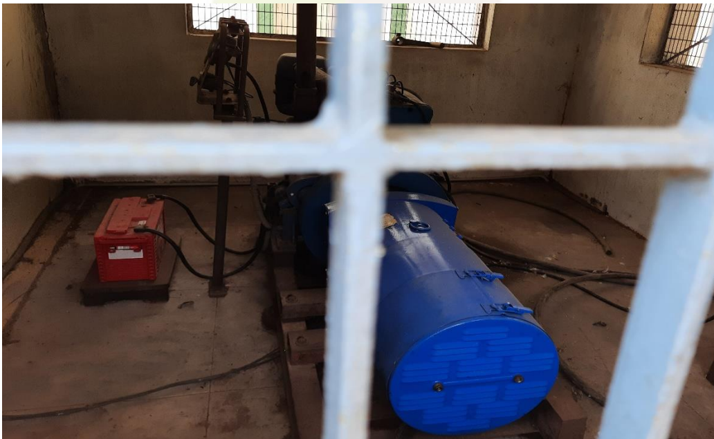
Hostel Diesel Generator
