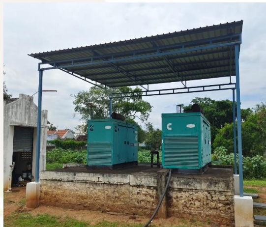
Shed for DG
